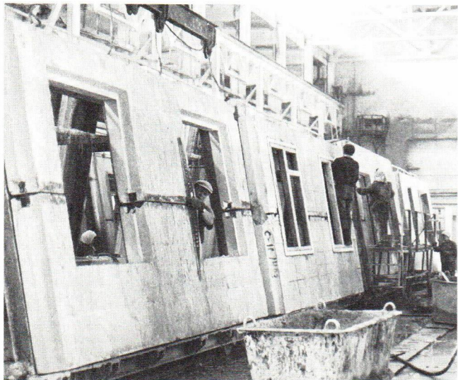
Finishing of the elevation panels, Obouchovsky, Leningrad Fertigung der Fassadenpaneele, Obukowskij, Leningrad Fabrication des panneaux de façade, Obouchovski, Leningrad
